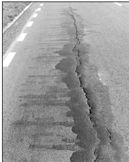
Fig. 4. Longitudinal cracks in the surface resulting from a non-uniform settlement of an embankment
